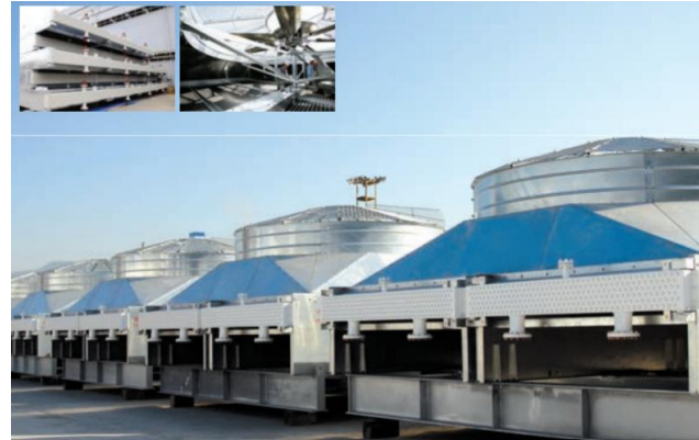
Air Cooled Heat Exchanger
